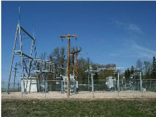
Image: Electrical substation
